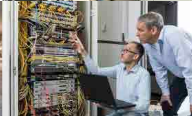
Stefan Kadoić, Jörg Horand perform a security check at the data center at BGE headquarters
