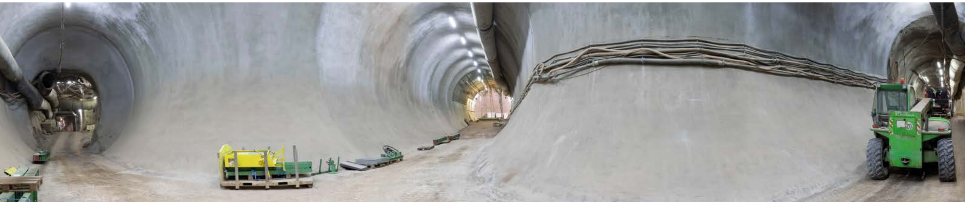
Konrad shaft mine: Drift crossing at the crusher plant, 2nd level
