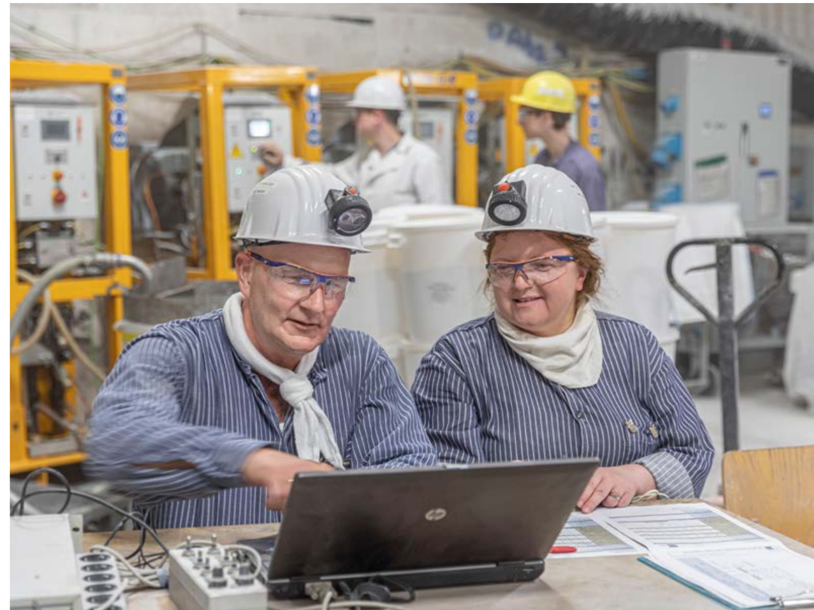
Asse mine: Injection work – adjusting the parameters for injecting a particle-reinforced injection medium to create a seal at the flow barrier SB-750-7 (750 m level); Horst Mentzel and Astrid Hofschlag (BGE TECHNOLOGY GmbH)
