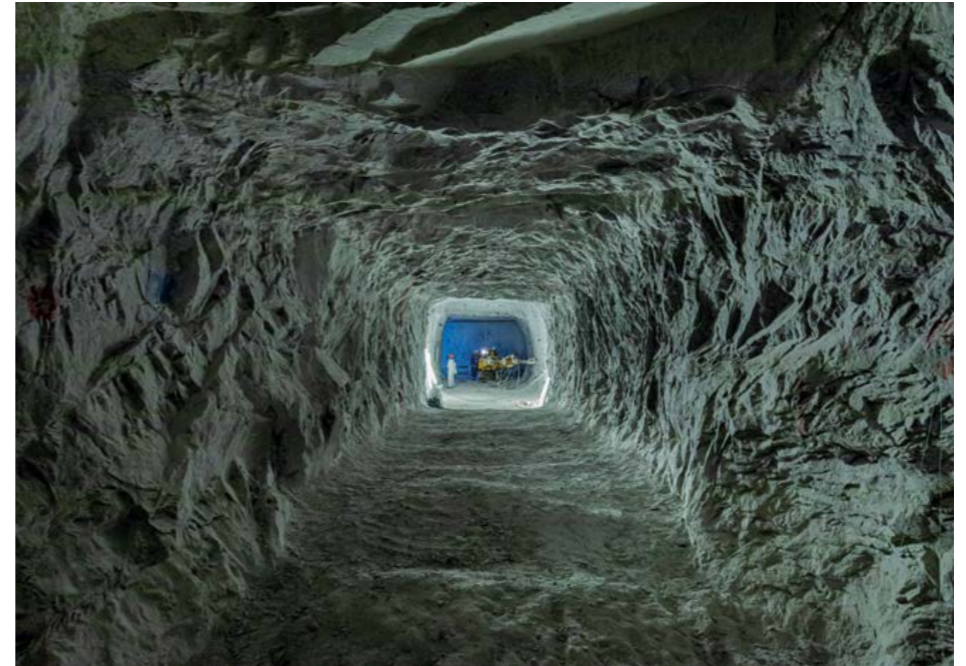
Morsleben repository: View from the excavated, 40 m long drift for the demonstration structure before re-cutting the contour
